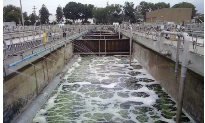
To increase water recycling at LAGWRP key modifications are in the planning stage such as providing additional equalization capacity.
